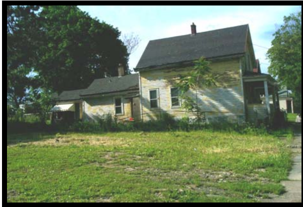
Figure 2: Dilapidated Housing in the Fruit Belt
